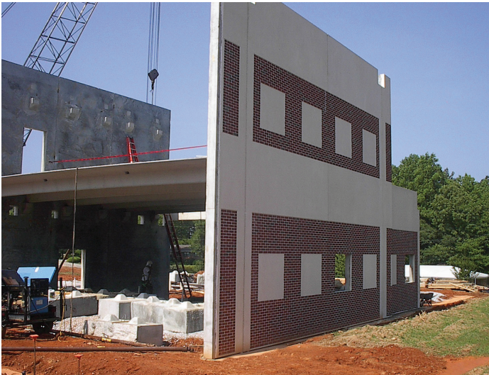
Precast concrete panels allow the building to be dried in before the floor slab is cast, which eliminates weather impacts and casting-related damage to floor slabs.
